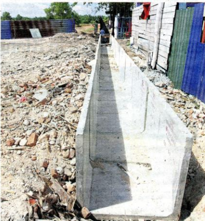
A new drain is being constructed along the fence of the factory.
